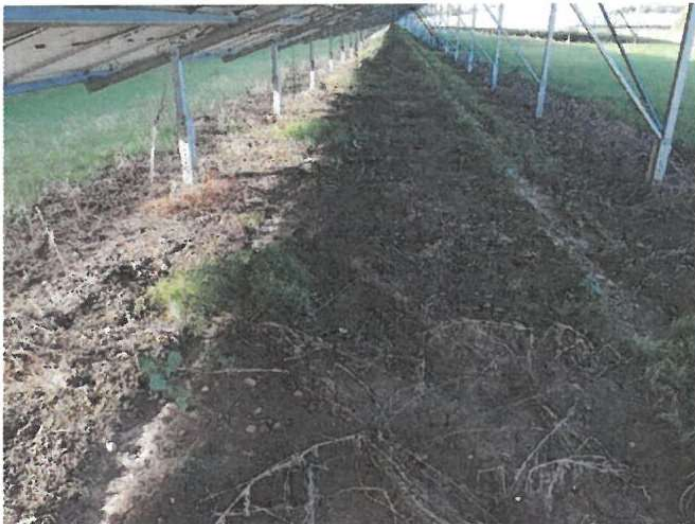
Figure 6: Channels created by panel runoff within 12 months of site operation commencing
